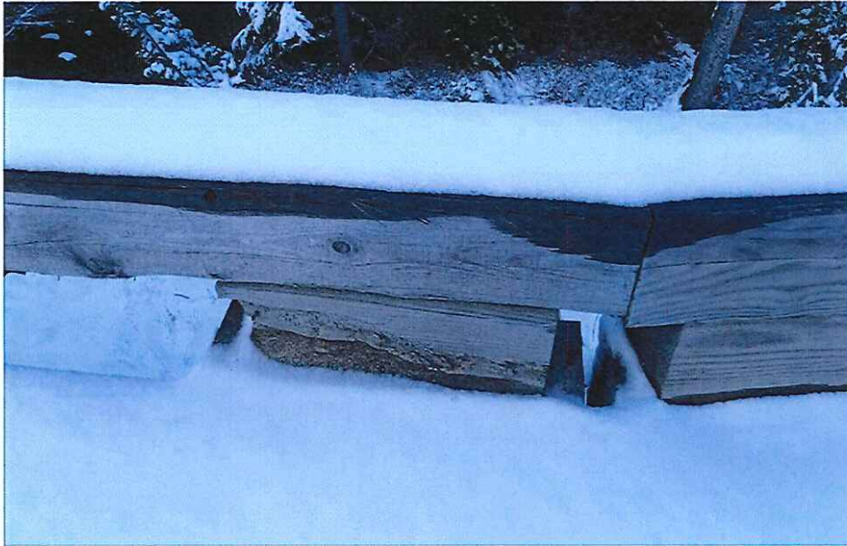
CK2362 Rotten guard rails
